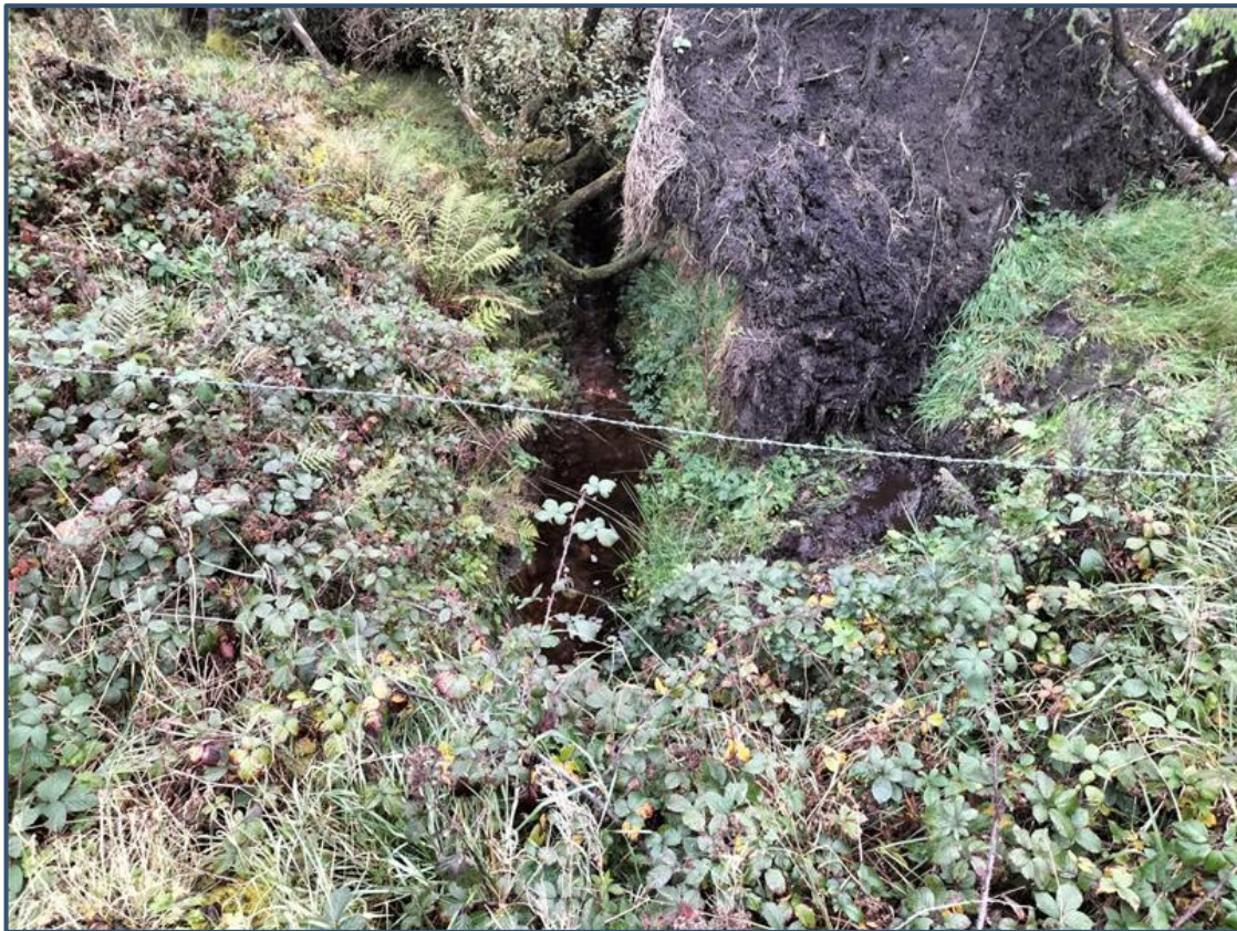
Plate 4-34. A representative image of survey location GCI, facing downstream from atop the culverted section.
